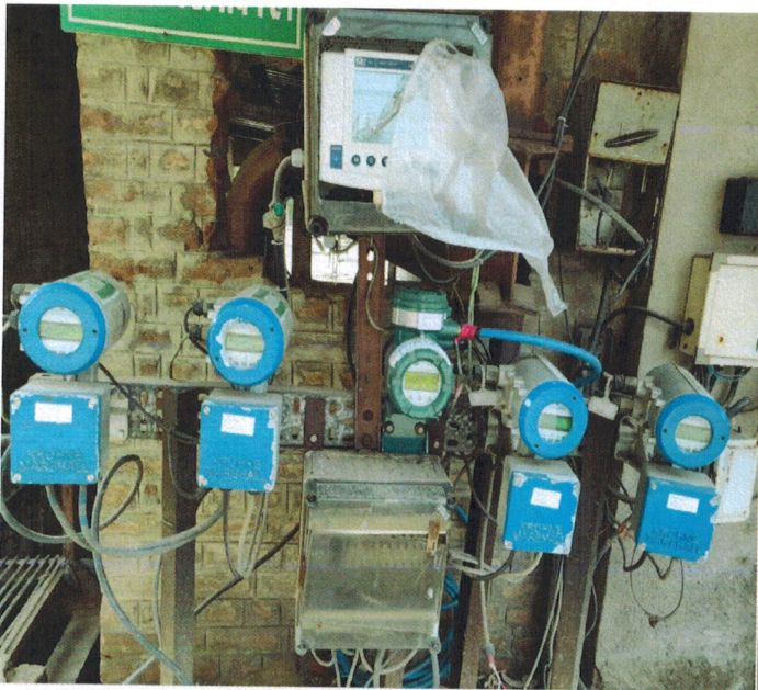
Flowmeters for Utilization of Treated Effluent for Irrigation
